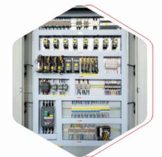
电控区域 Electrically controlled area
